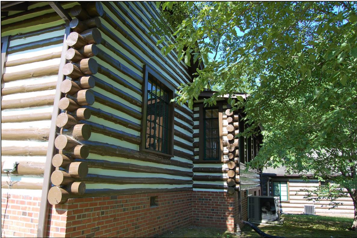
Figure 16. Detail of north rear elevation of Morgan house with projecting sunroom at center
