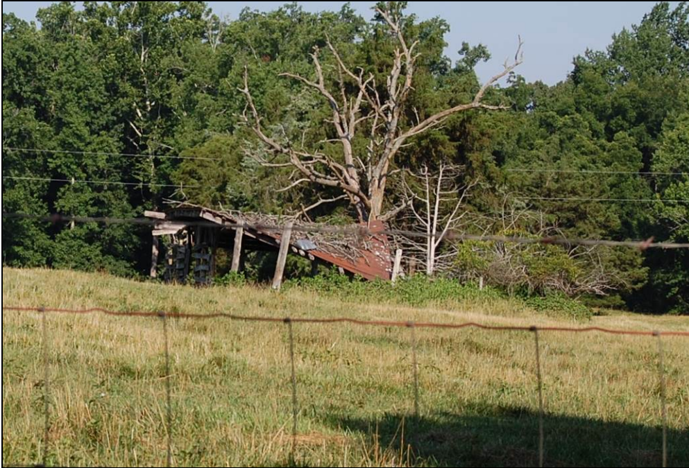
Figure 29. Looking west at ruinous run-in shelter
