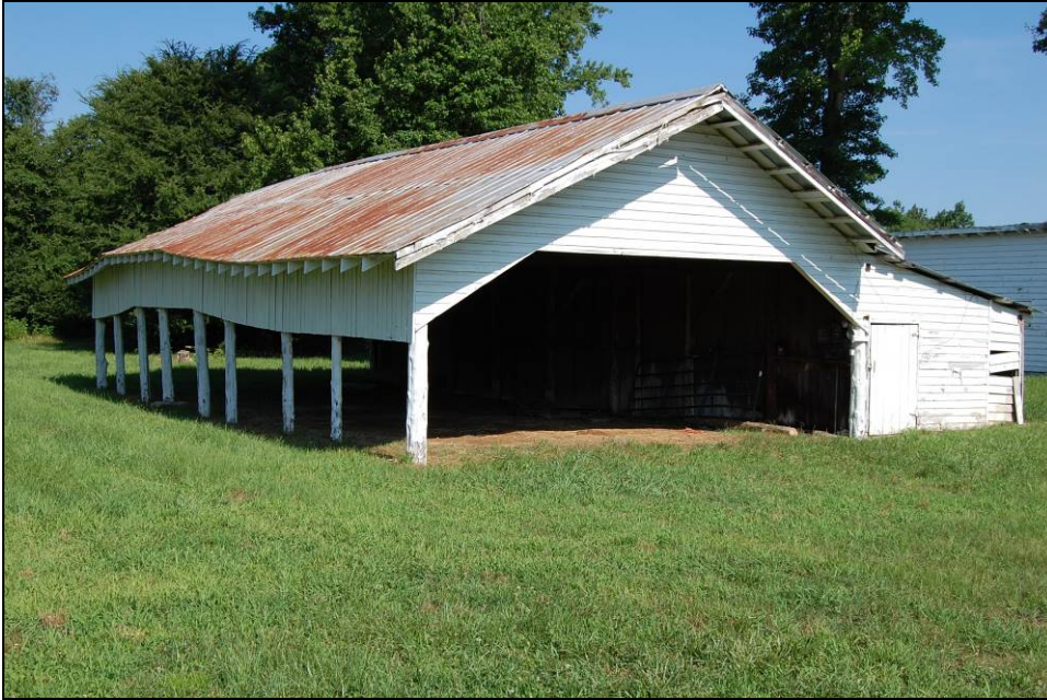
Figure 25. Long south and gable-end east elevations of equipment shed with milkhouse at right distance
